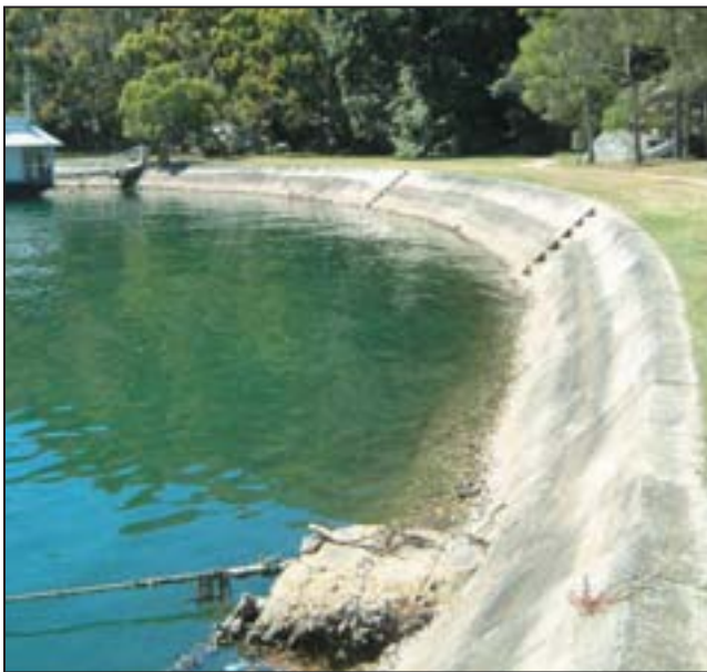
Above: The steep, blank face of the seawall at Pearl Bay does not provide habitat for intertidal life.
