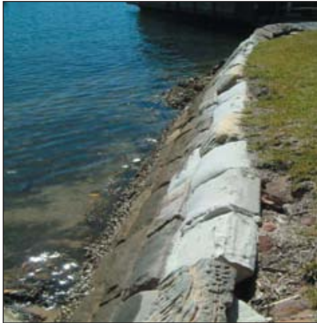
Above: Seawalls at Pearl Bay, which will be the site of an upcoming restoration project.
